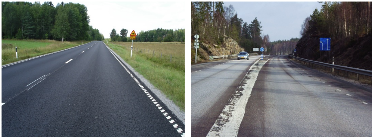
Figure 1 Brand new road markings (left) and road markings showing damage from the plough (right).
