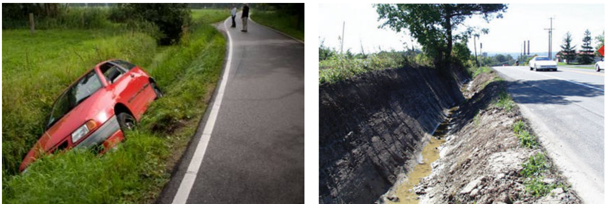
Figure 13: Examples for hazardous roadside ditches (Source: [B.8])
