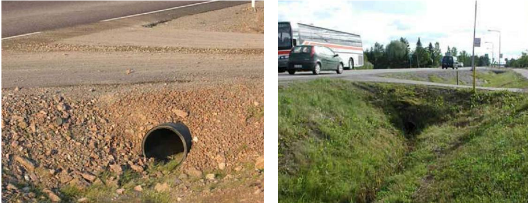
Figure 11: Examples for hazardous drainage features (Source: [A.2])
