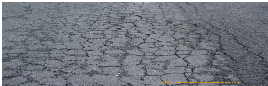
Fig. 7: Alligator Cracking in Asphalt Concrete (from WALT infrastructural Services Ltd).
