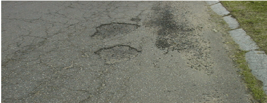
Fig. 9: Ravelling of an Asphalt Pavement (from http://www.pvpc.org/web-content/graphics/images/trans/pave_gif/surf_wear.gif ).
