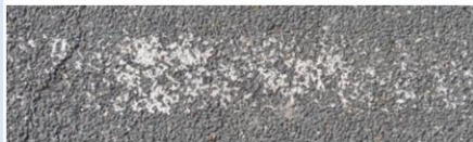
Figure 57: Old road marking with time wear
