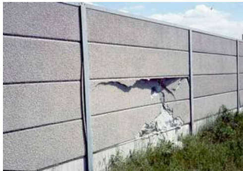
Figure 39: Damaged noise barrier
