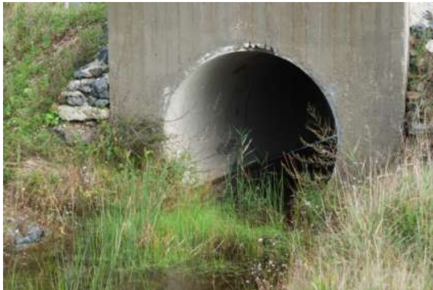
Figure 7-1 A culvert used by Fire-bellied toad ( Bombina orientalis ) to cross a highway in Hungary (Photograph Dennis Wansink).
