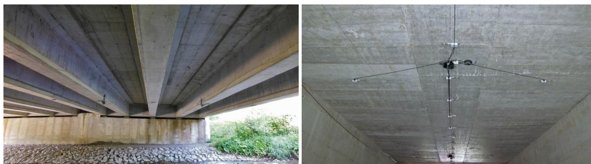
Figure 11: Typical SiWIM ® installations in Slovenia
