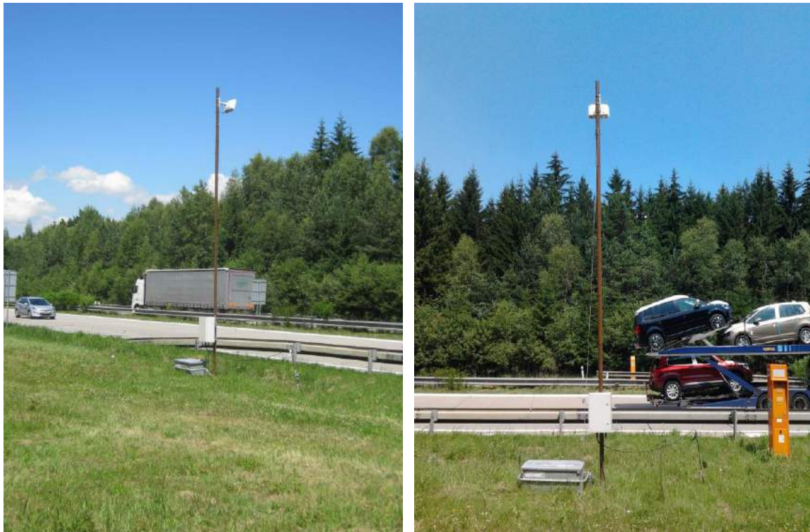
Figure 16: Wavetronix detector as installed on section 4
