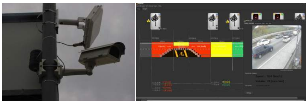
Figure 3: Portable traffic detectors (left) and controlling software of portable control system ViaZONE, which was developed and pilot tested on motorway D1 in 2013
