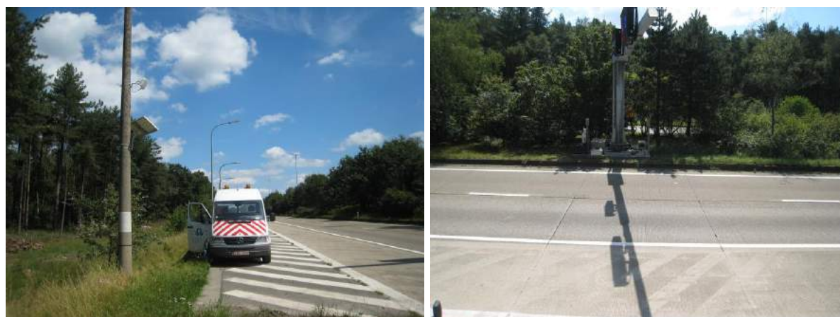
Figure 40: BRRC Wavetronix Smartsensor HD (digital wave radar) at KP 23.20
