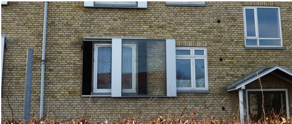
Figure 5.5: Extra movable noise protection placed in front of existing living room window. No noise protection has been applied to the kitchen window.
