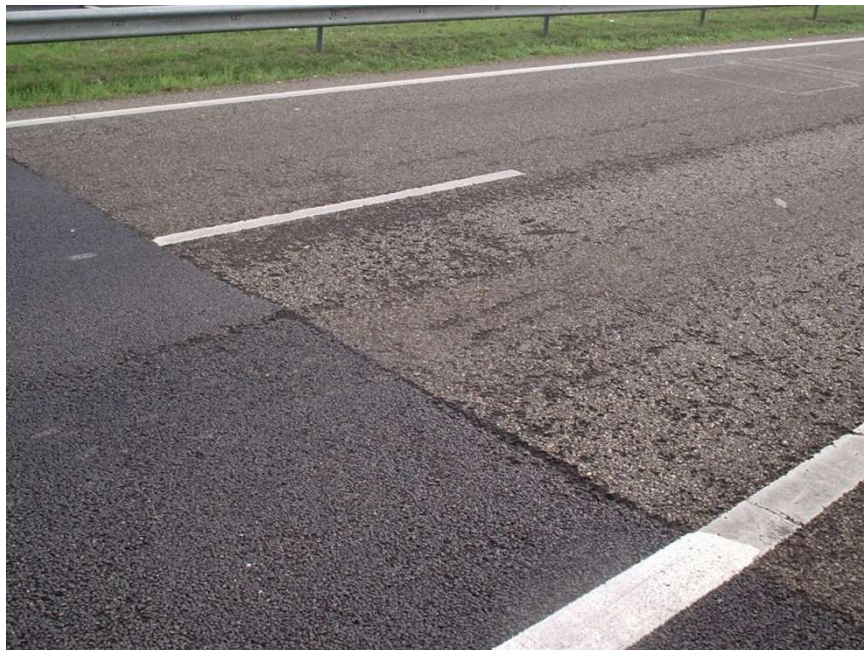
Raveling at the end of an inlay
