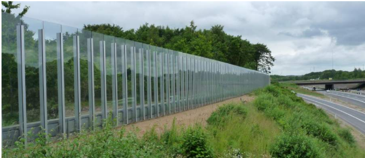
Figure 3.16: A transparent noise barrier along a motorway.
