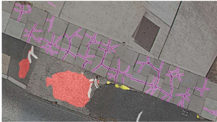
Figure 6: Identification of sidewalk defects using AI.
