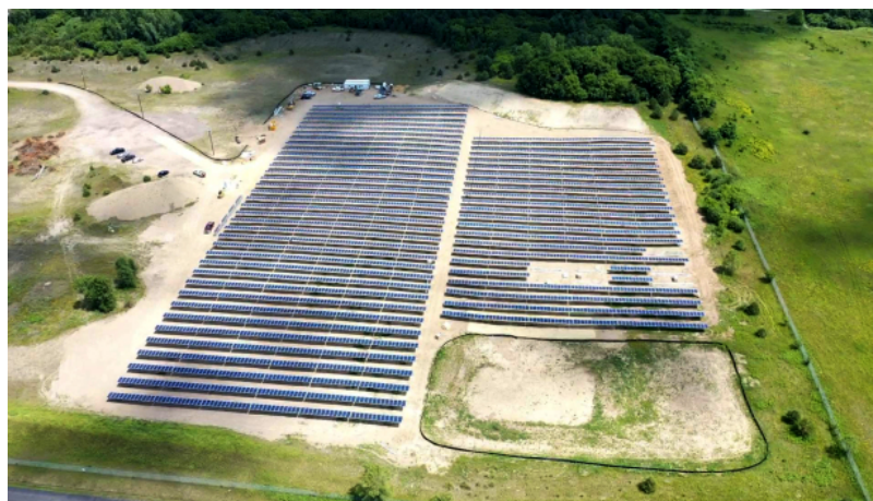
Figure 88.- Solar Garden in Afton (Minnesota). Source: MnDOT (2020)
