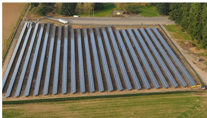
Figure 85.- Baldock Solar Station at a safety rest area in Oregon. Source: Innovative (2021)
