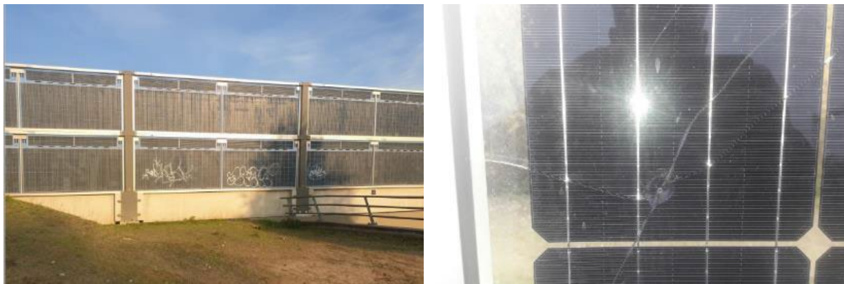
Figure 100.- Vandalism events on the PVNB in Uden. Source: SH Final (2020)
