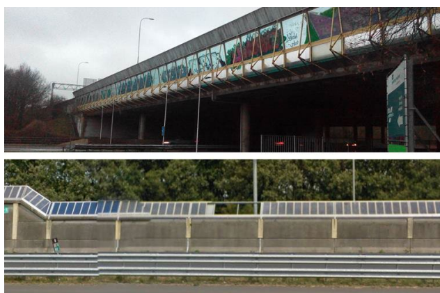
Figure 97.- Several modules missing at the PVNB along the A27 highway. Source: SEAC (2015)
