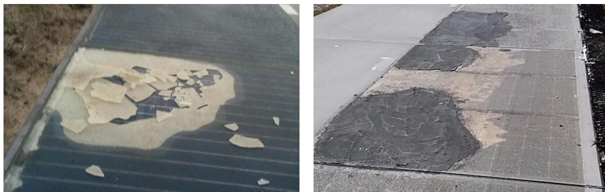
Figure 95.- Damage to the SolaRoad in Krommenie, The Netherlands. Source: deorkaan (2015)
