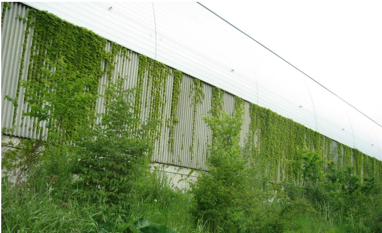
Figure 134: Greenery covering the lower part of a high noise barrier.
