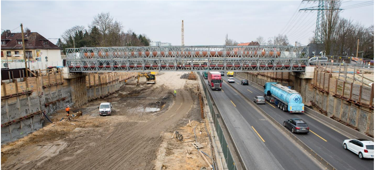
Figure 140: Situation during construction phase – traffic shifted to one side and speed limits.
