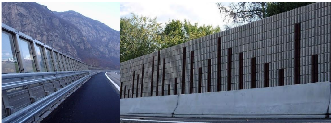
Photos: Different types of integrated noise and safety barriers of different materials in Europe (steel & transparent left side and fully concrete type right side).
