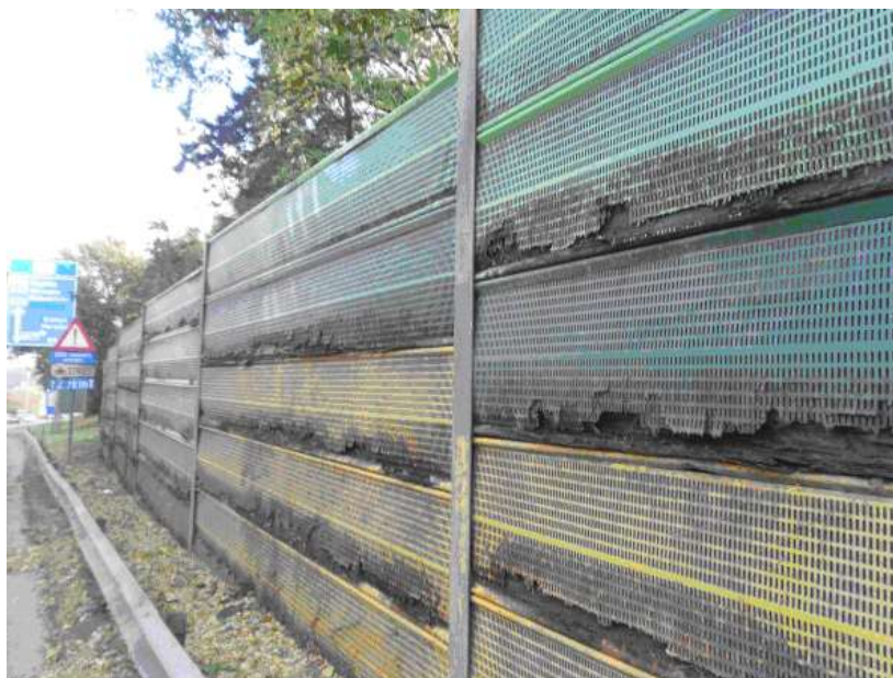
Figure 3: Example of a noise barrier with evidence of significant degradation
