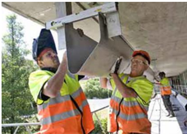
Figure 11: Gutters made out of stainless steel are mounted under a bridge across Lake Mälaren, the main drinking water source for the Stockholm region (photo: Swedish Transport Administration)
