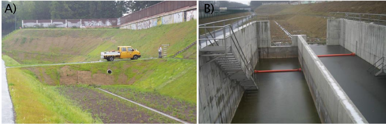
Figure 21: Example of German treatment facilities. A) Infiltration pond. B) Sedimentation tank followed by an infiltration step (soil filter) (photo: BASt/DEGES)
