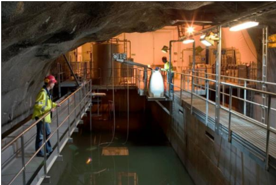
Figure 18: Sedimentation basins inside the Södra Länken tunnel in Stockholm. The containers in the background are made out of stainless steel and contain the flocculent. An oil skimmer is visible just beneath the water surface (photo: Swedish Transport Administration)
