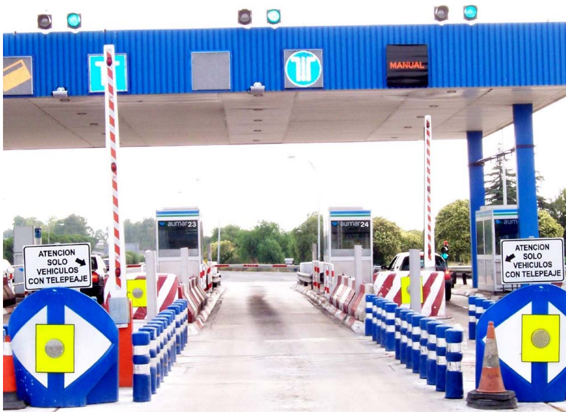
Motorway toll collection point in Spain (Playas de peaje de la Autopista de San Juan. Aumar)
